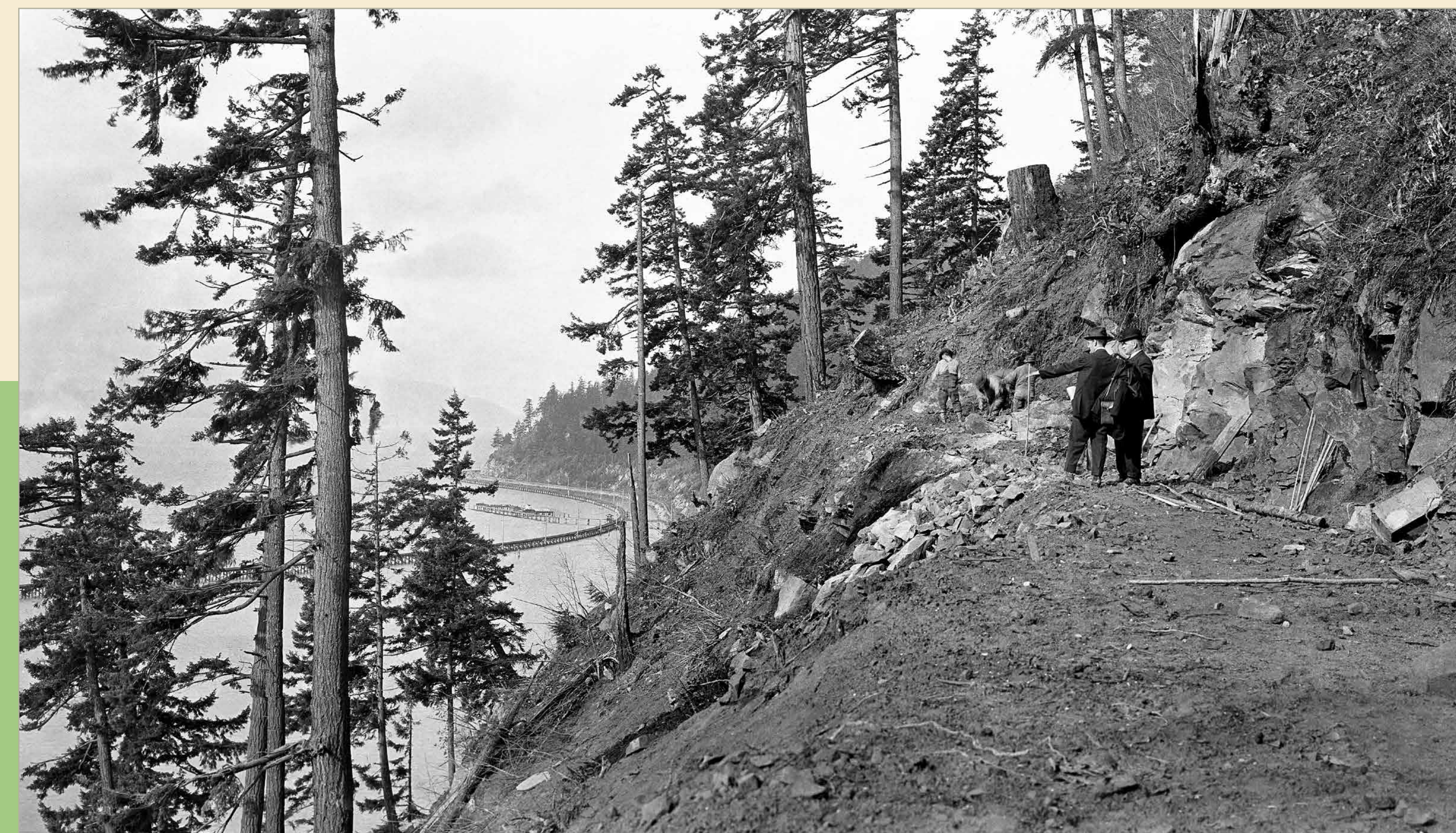
Cyrus Gates (right) out checking progress on the construction of Chuckanut Drive, circa 1914. The State's use of convict labor on the project in 1910 had been a failed experiment. Prisoners had little incentive for breaking rocks in the hot sun and laborers were hired from then on.
